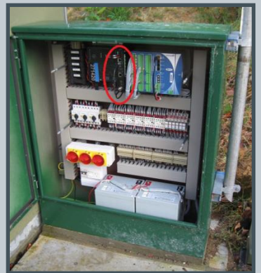
Aprisa SR in roadside cabinet
