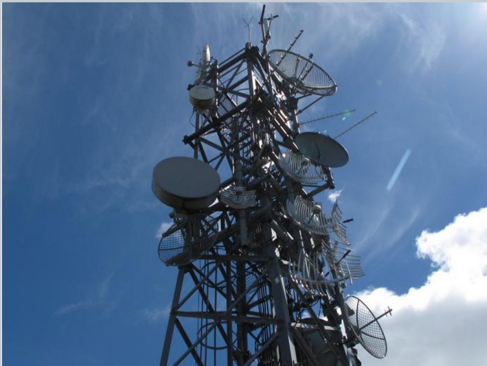
CHORUS TE UKU TOWER USED BY WEL NETWORKS UNDER A CO-SITE AGREEMENT
